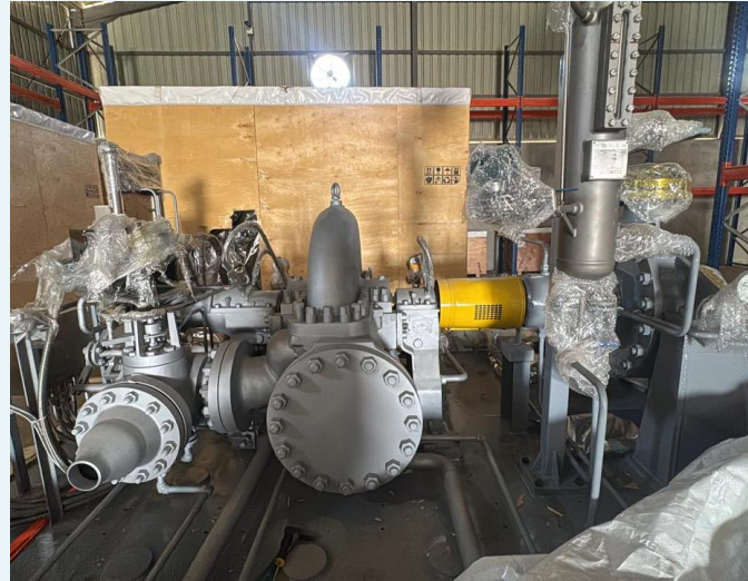
INTEGRATED PIPING & VALVES
