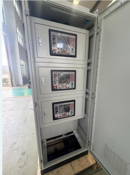
LOCAL CONTROL PANEL
